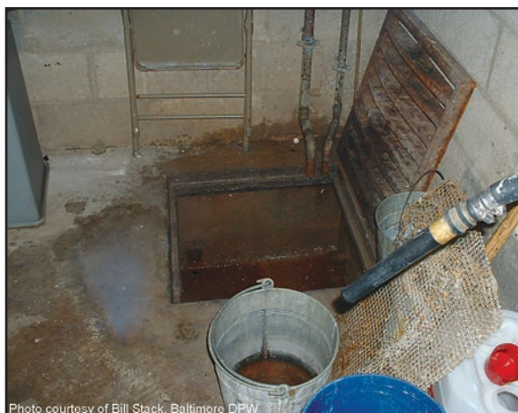
Figure 3: A common industrial cross connection is a floor drain that is illicitly connected to a storm drain
